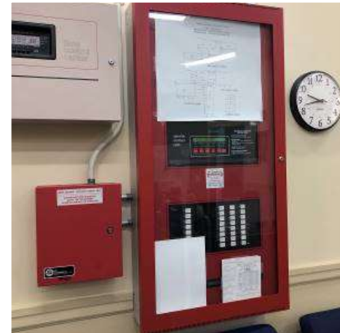
The fire alarm system does not meet current regulatory requirements
