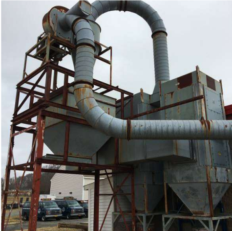
Shop dust collectors require explosion isolation dampers, spark detection and spark arresting equipment
