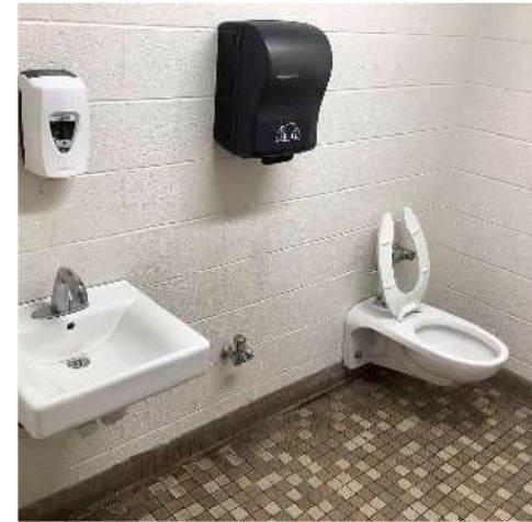
AAB Non-Compliance: Multiple toilet rooms lack maneuvering clearances and assist devices
