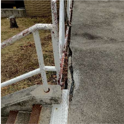
Roof at loading dock corridor deteriorating
