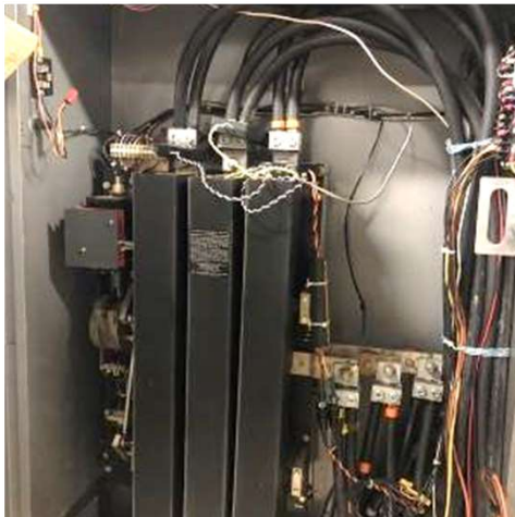
Emergency power system in poor condition
