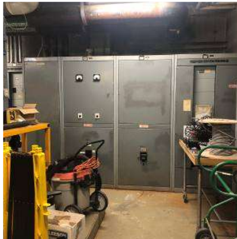
Normal power system in poor condition
