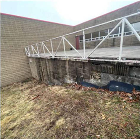
Water damage at exterior patio
