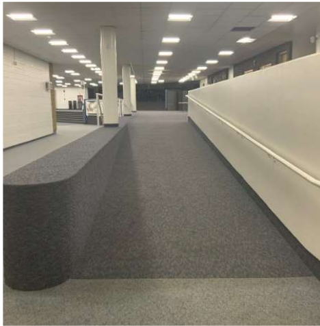
AAB Non-Compliance: Public ramps too steep, lack compliant handrails, typical for all
