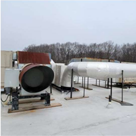
Energy recover units, serving kitchen, culinary arts and bakery, have deteriorated beyond repair
