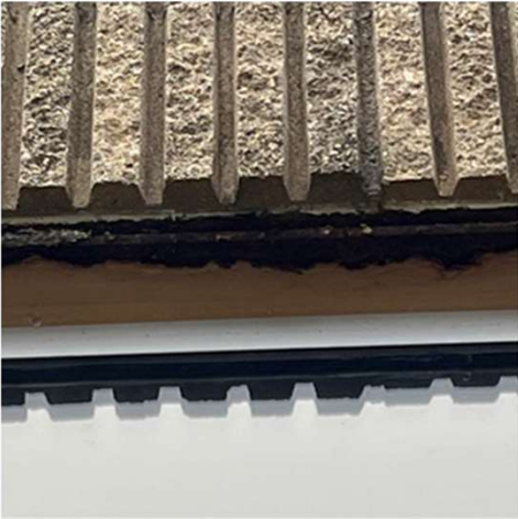
Lintels at masonry opening corroded and require replacement
