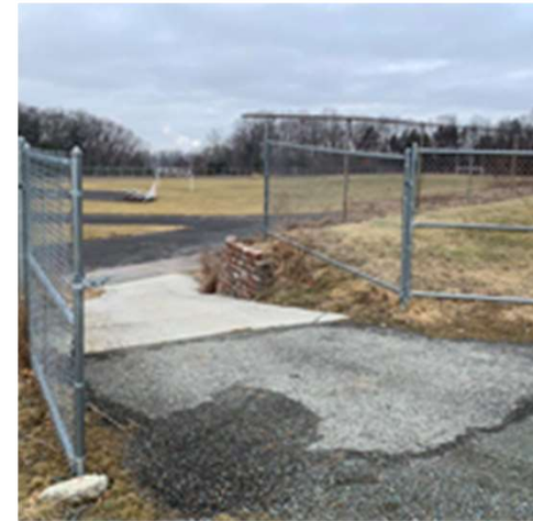
Fields, bleachers and the press box AAD non-compliant
