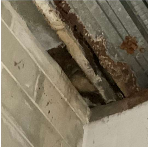
Damaged metal deck due to water infiltration from exterior patio above
