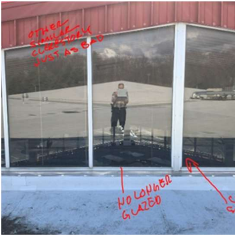
Glazing at storefronts brittle cracking and in many cases missing, glazing film at all instances hazy, cracking and peeling
