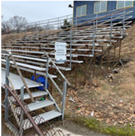
Athletic field conditions are fair to poor, the track is visibly deteriorated
