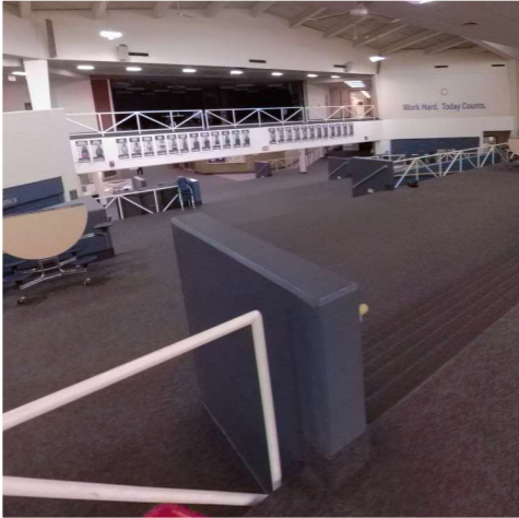
Guardrails at mezzanines and stairs not code compliant
